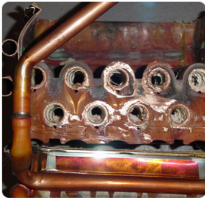
Scale build-up in the heat exchanger tubes of a tankless water heater without EasyWater treatment.
